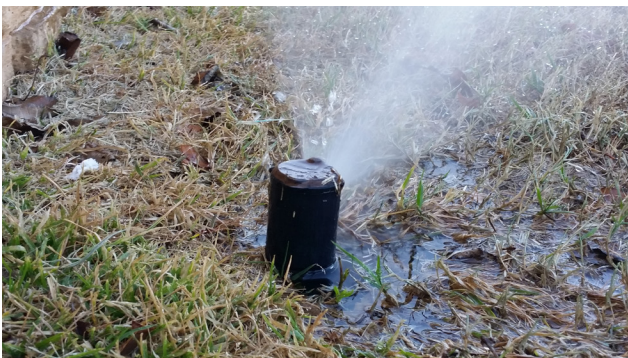
Figure 4. Sprinkler head leaking and causing ponding at the base.
