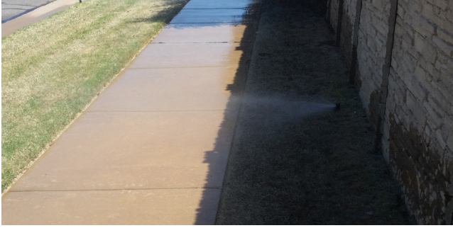
Figure 1. Sprinkler head spraying a sidewalk.
