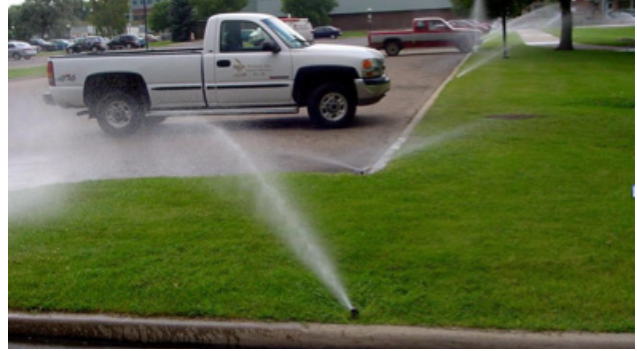
Figure 5. An irrigation zone with a mix of rotors and fixed spray sprinklers.
